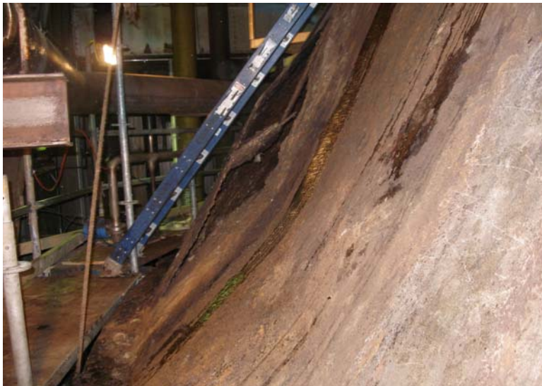
Cone Failed from Buckling, Cracking, & Corrosion
